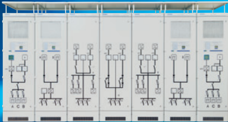
水力发电设备的内部电源 Internal power supply of a hydrofacility
