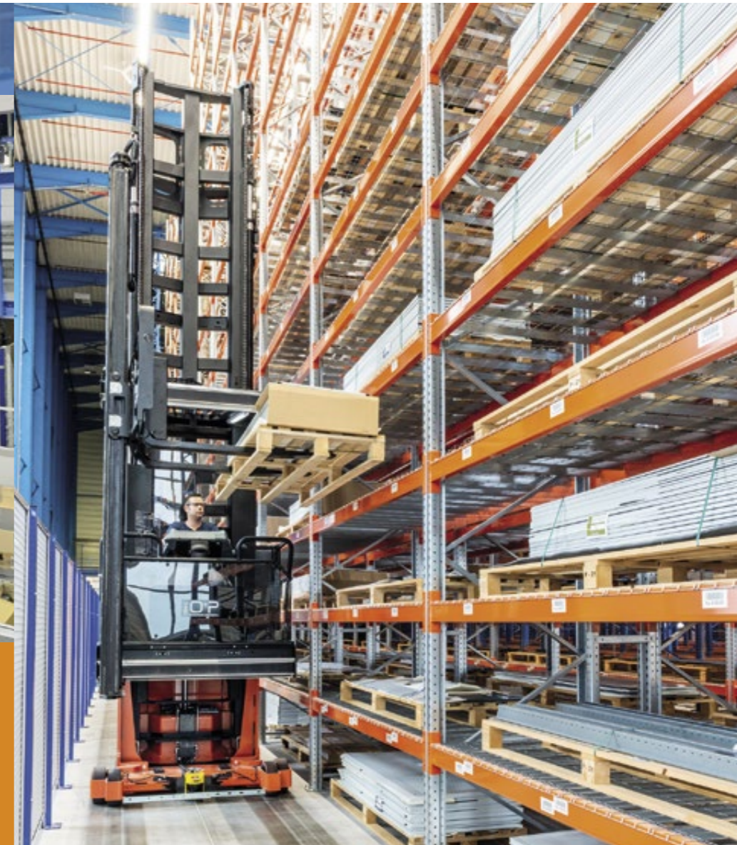
Narrow-aisle store for special-pallets with a drop height of up to 16.50 m
