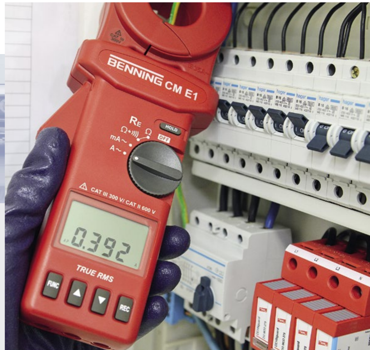
Measuring the total leakage current in a sub-distribution system.
