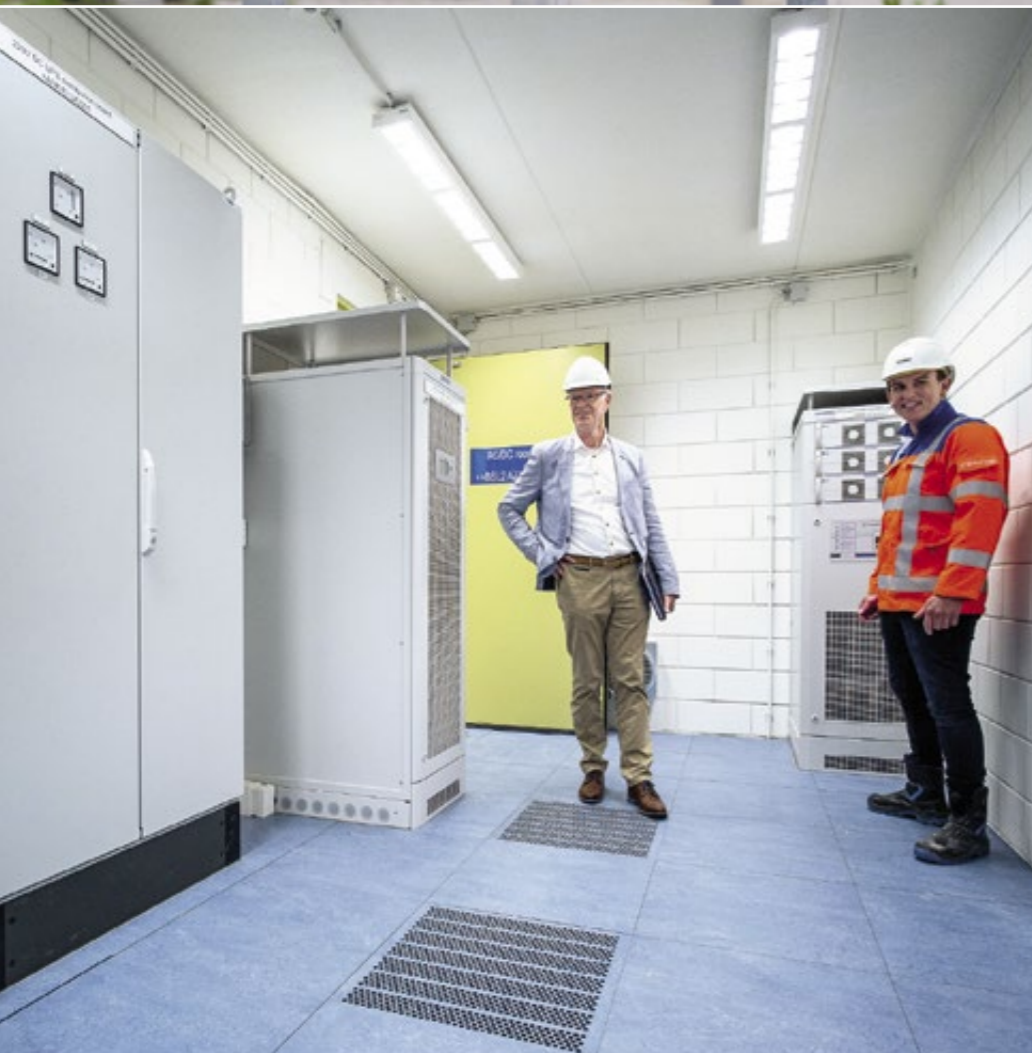
A view of the Borssele high-voltage substation in the process of inspection. The substation is protected from grid disruptions or failures thanks to two ENERTRONIC modular SE UPS systems (each one comprising 60 kW) together with two BENNING rectifier systems (220 VDC / 200 A) (see background).
