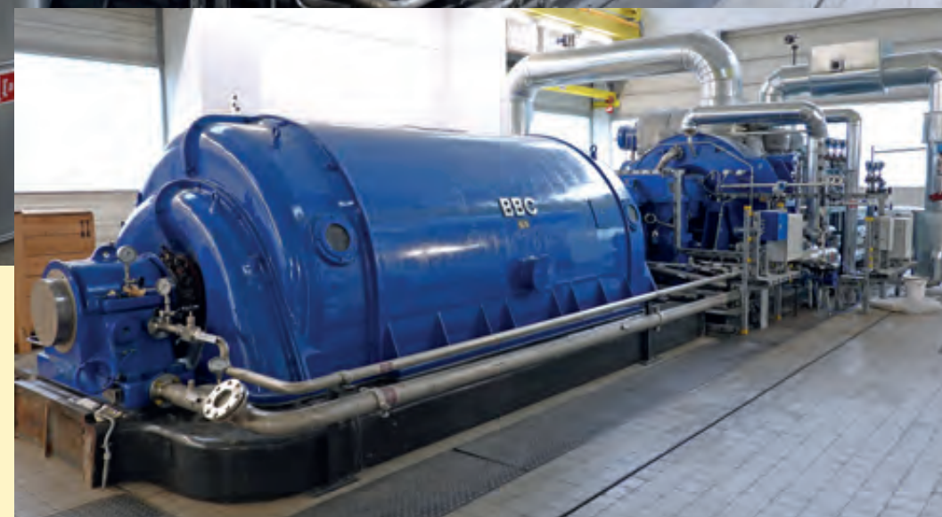
The three steam turbines, some of which are over 50 years old, were modernized in 2018 and brought up to the current state of the art
