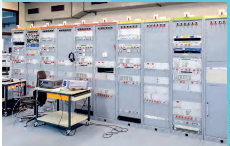
(below) View into the technical rooms of the transmitter
