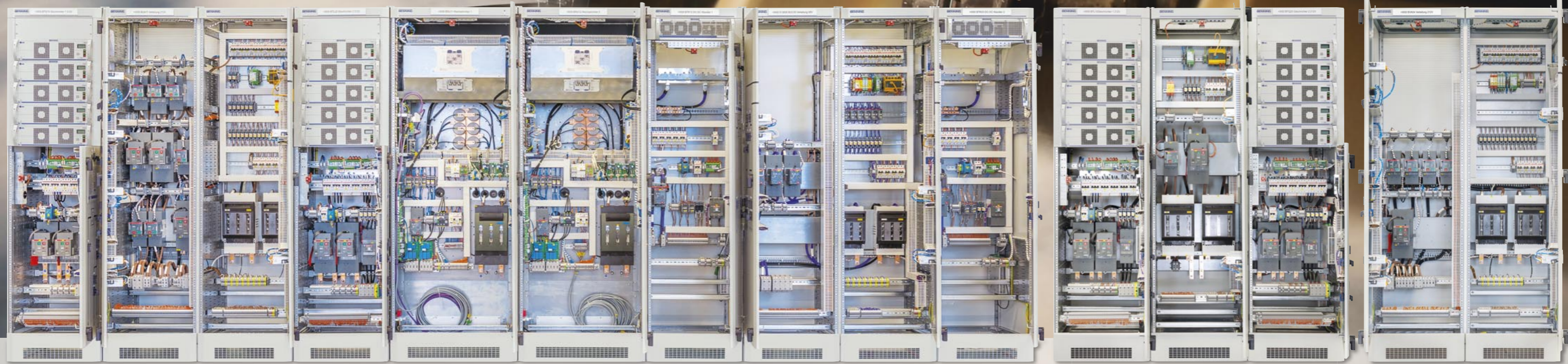
Thanks to motorised output switching in the distribution systems supplied by BENNING, there's fully automated management of operations from the control console at all of the power stations' system-related voltage levels
