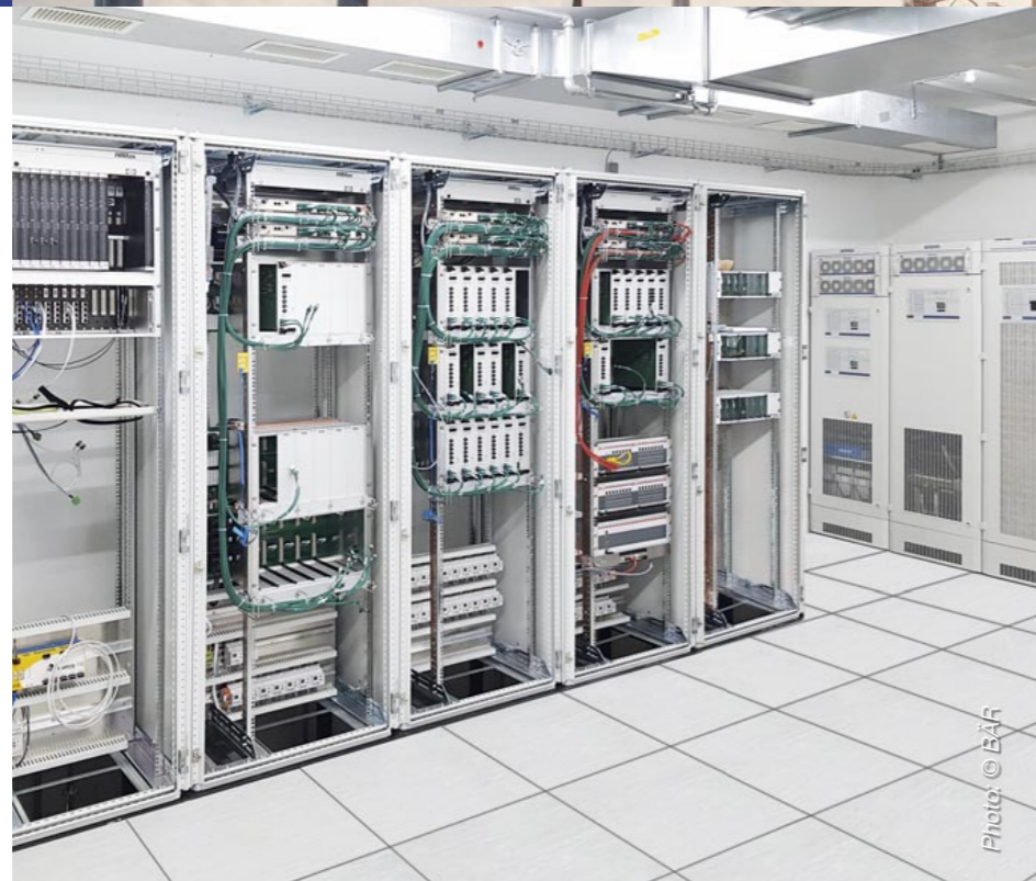
Here's a look inside the new Montbovon interlock system plant during the process of installation. BENNING's EUROLOCKING® power supply system (illustrated in the background) protects the heart of the interlock system, the PLC control system, against grid faults.
